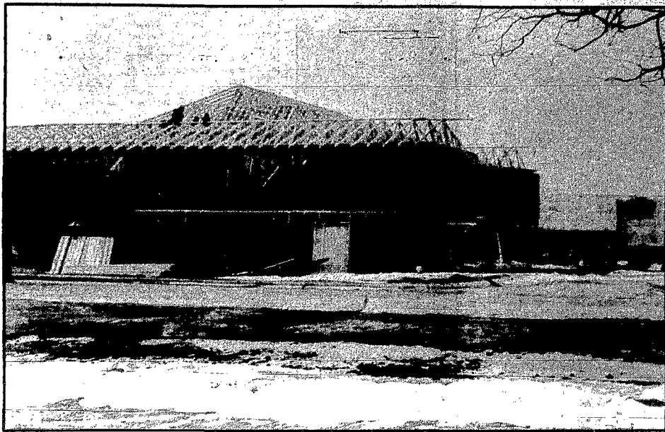
THE NUMBER OF BUILDING permits recorded in Wayne this year is expected to top last year's total. However, the total volume of construction will be less than a year ago. Above is one of two apartment buildings under construction just south of El Toro. Total project cost of these is expected to be about $440,000, the largest project this year.
